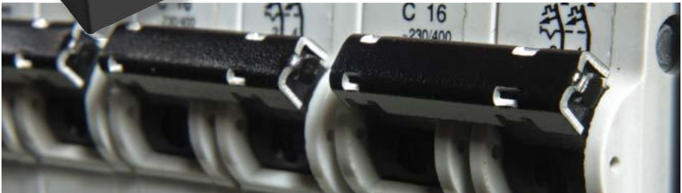
Two open frame solenoids drive a change over switch
